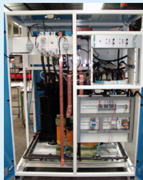
Rectifier for particle accelerator
